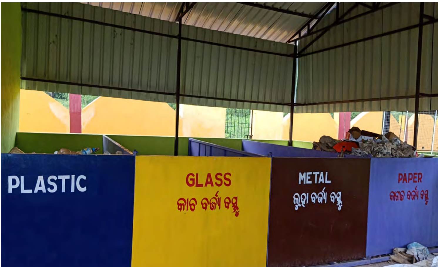
Chambers for secondary segregation of non-biodegradable waste in MRF
