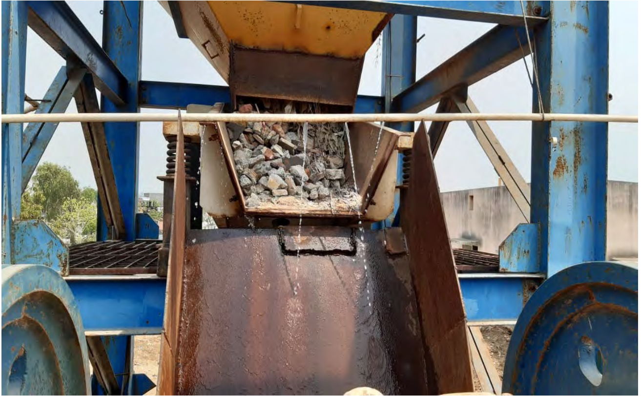
C&D waste processing facilities in Vijayawada
