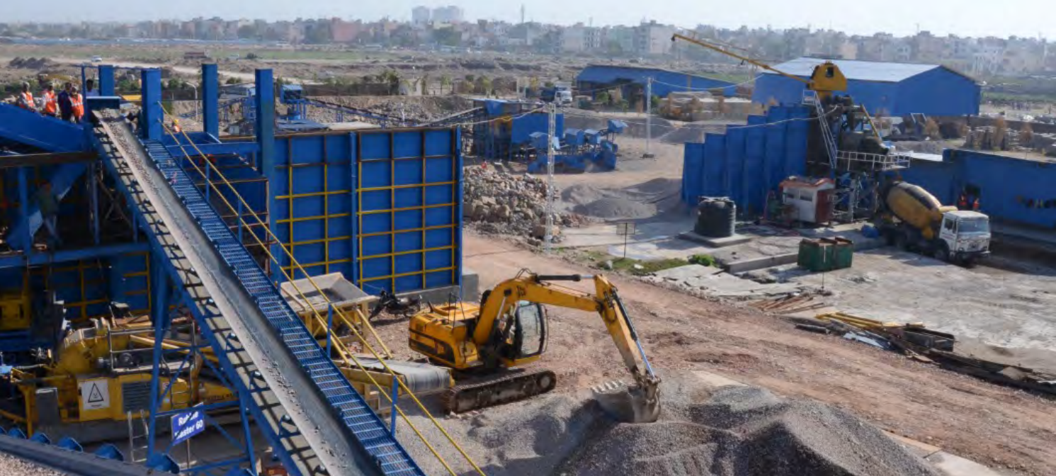
C&D waste processing plant, Burari
