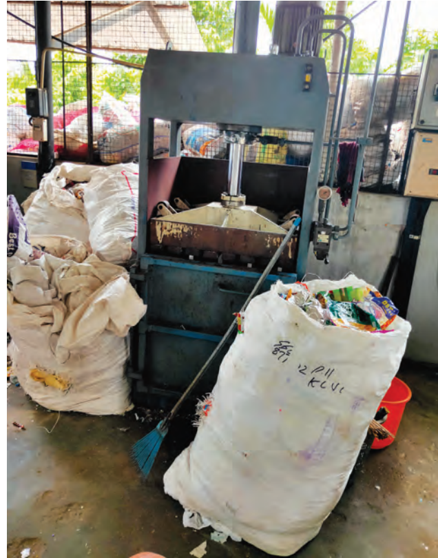
Baling machine inside a material recovery facility
