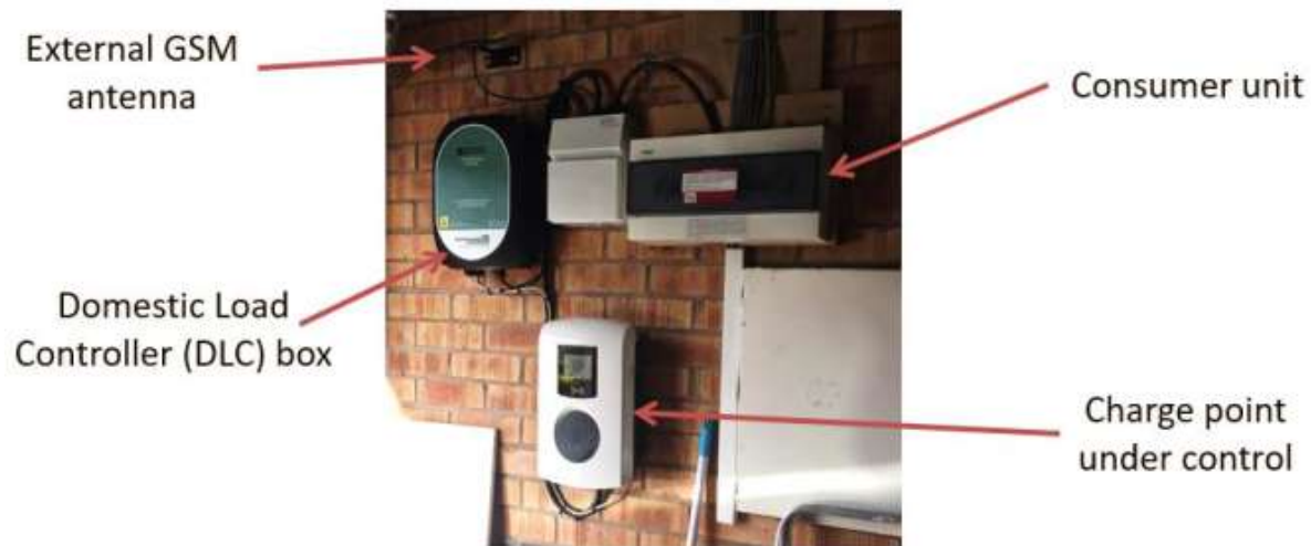
Figure 2.20: Typical example of the EV charge point and DLC installation in customers' homes ( LV Connect and Manage Closedown Report, 2019 )
