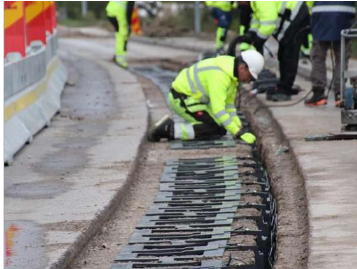
Figure 9.9: Installation of coils for wireless energy transfer in the Smartroad Gotland pilot ( Smartroad Gotland , n.d.)
